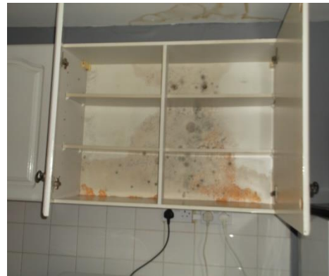
Penetrating damp to kitchen wall and ceiling
