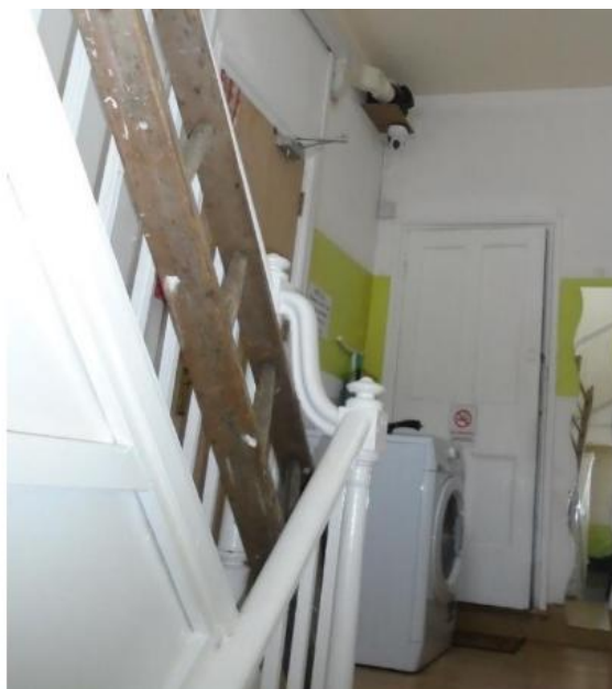
Washing machine located on escape route
