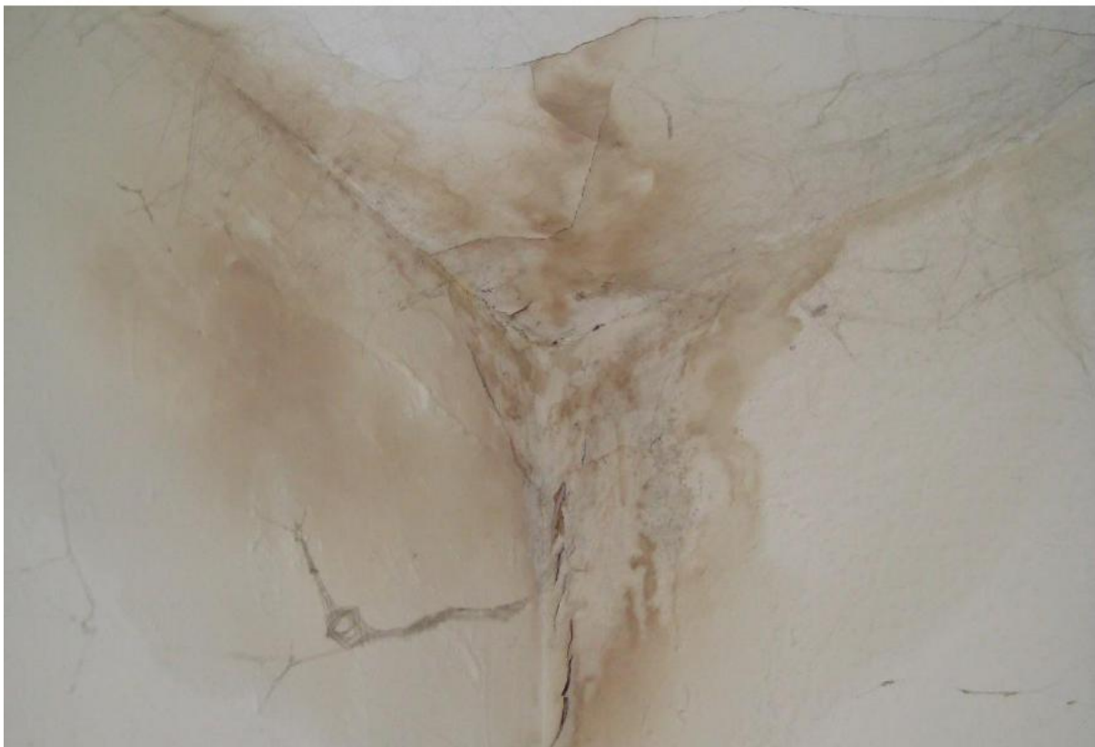
Damp penetration from leaking shower
