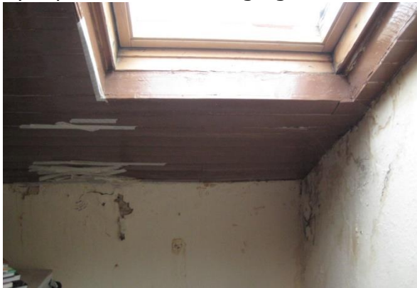
Leaking roof around roof-light in bedroom
