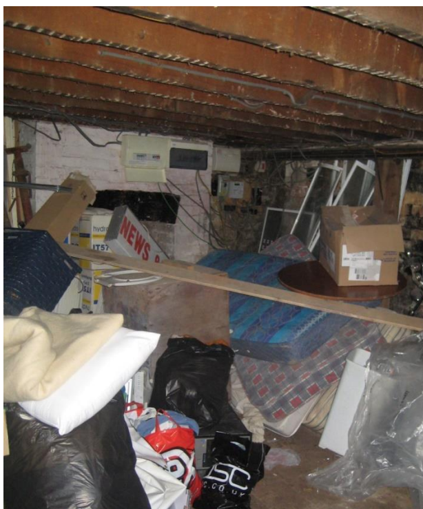
Accumulation of combustible material in cellar
