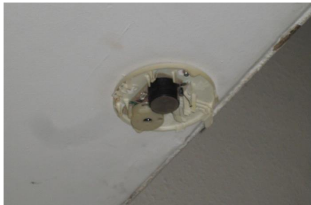
Defective smoke detector
