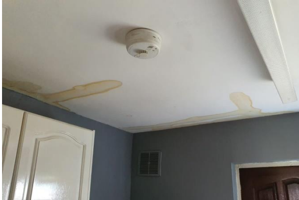
Penetrating damp to lounge ceiling
