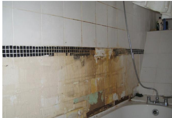
Damp and insanitary wall tiling
