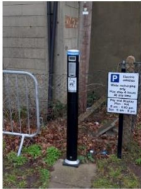
3kW charging point
