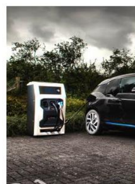
Rapid 50kW charger
