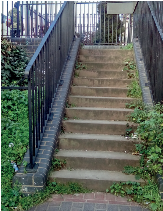
Poor access Leamington Spa
